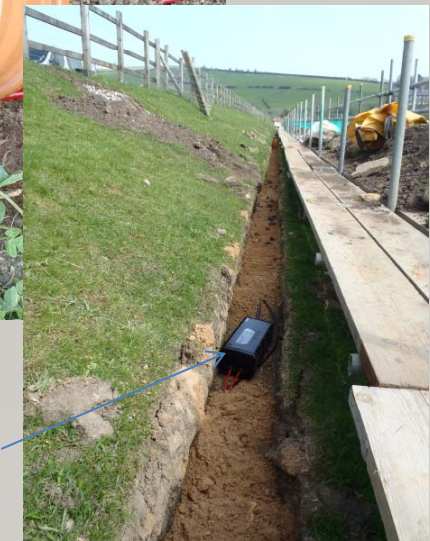
splice protection box
